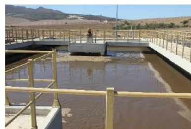
Reactor: Anoxic zone with two mixers
