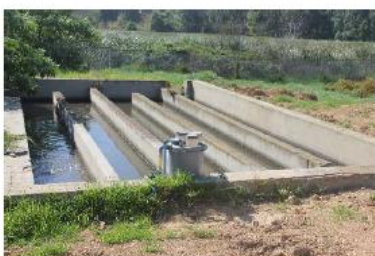
Chlorine contact channel
