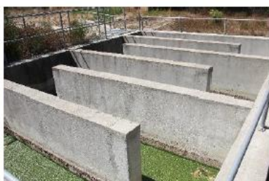
Chlorine contact channel
