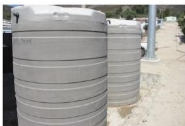
Three Aeration Tanks
