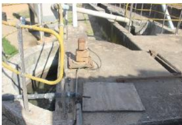
Inlet structure: Two vortex degritters
