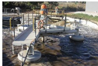
Reactor: Floating aerators
