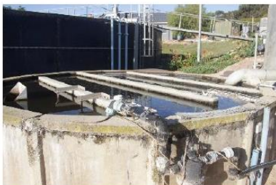
Chlorine contact tank
