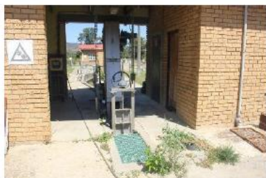
Inlet Structure with mechanical screen
