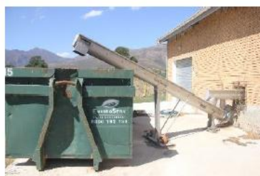
Dry sludge conveyor system (Huber)
