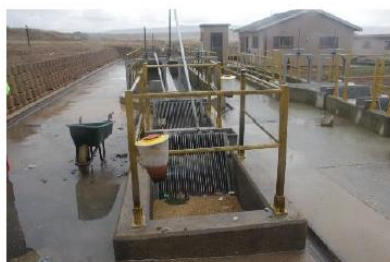
New Inlet works with 2 hand raked screens
