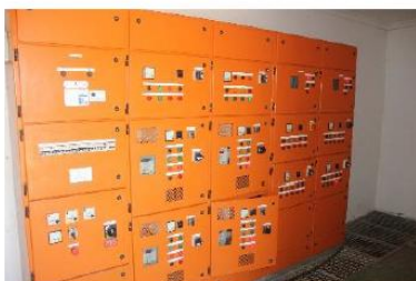
MCC for plant
